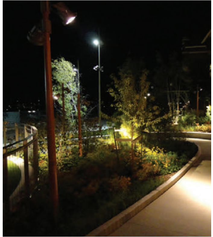
Site lighting along a pedestrian pathway. (Image Credit: Brook McIlroy)
