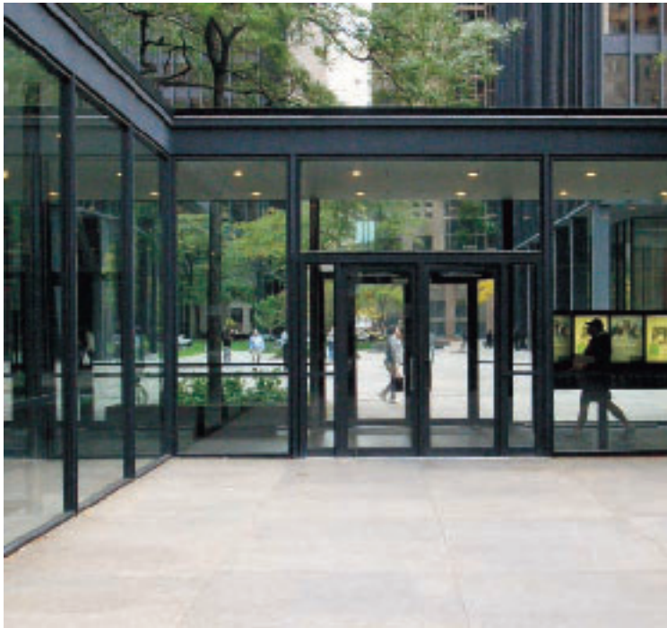
Hazard: Linkways are especially dangerous to birds as they will attempt to reach the habitat located beyond the glass. Glass treatments are strongly encouraged for these elements. Photo: FLAP
