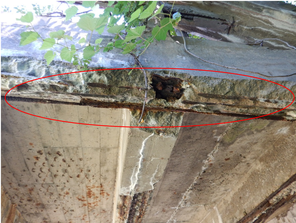
Bottom Chord, frost damage and spalling, with rebars and hangers exposed
