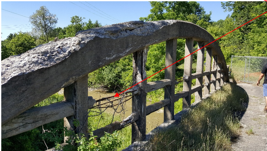
Failed rail with rail rebar exposed along South Arch
