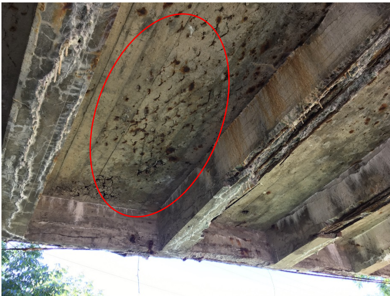
Rust stains visible at the underside of deck slab, indicating corrosion of the deck slab mesh reinforcing
