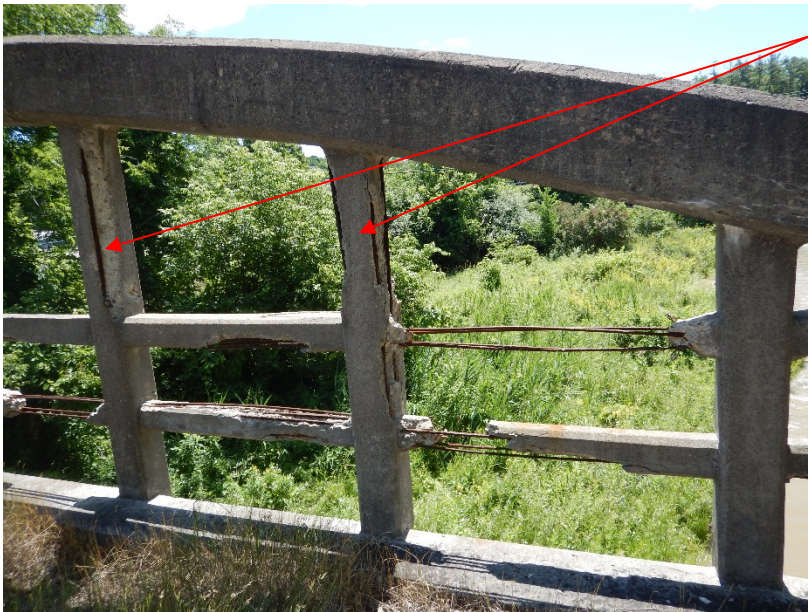
Loss of concrete cover to the vertical hanger steel as a result of spalling
