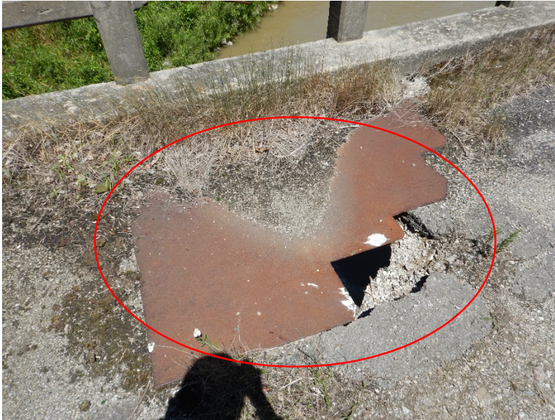
Large hole in the west end of deck, partially covered with a steel sheet.
