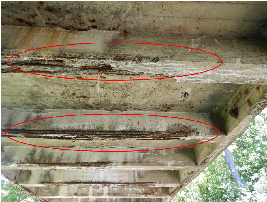
Floor beam with exposed and fully corroded rebars
