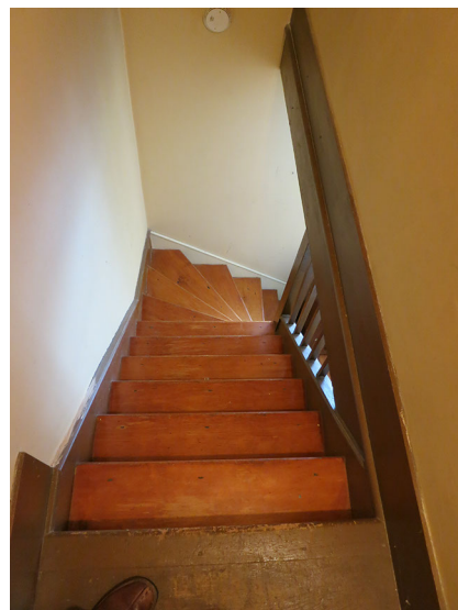
WCH-71 Attic stairs
