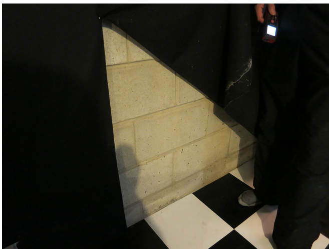
VKH-70 Basement concrete block
