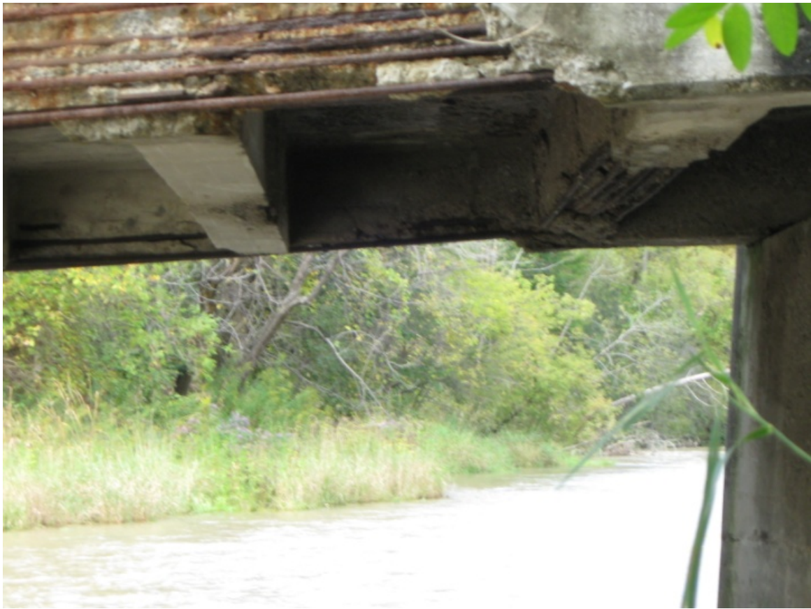
Photo 3 Cross Beams showing spalling
