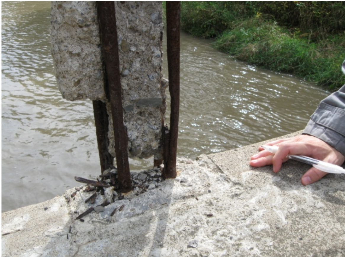
Photo 6 Vertical Spandrel Member showing severe spalling
