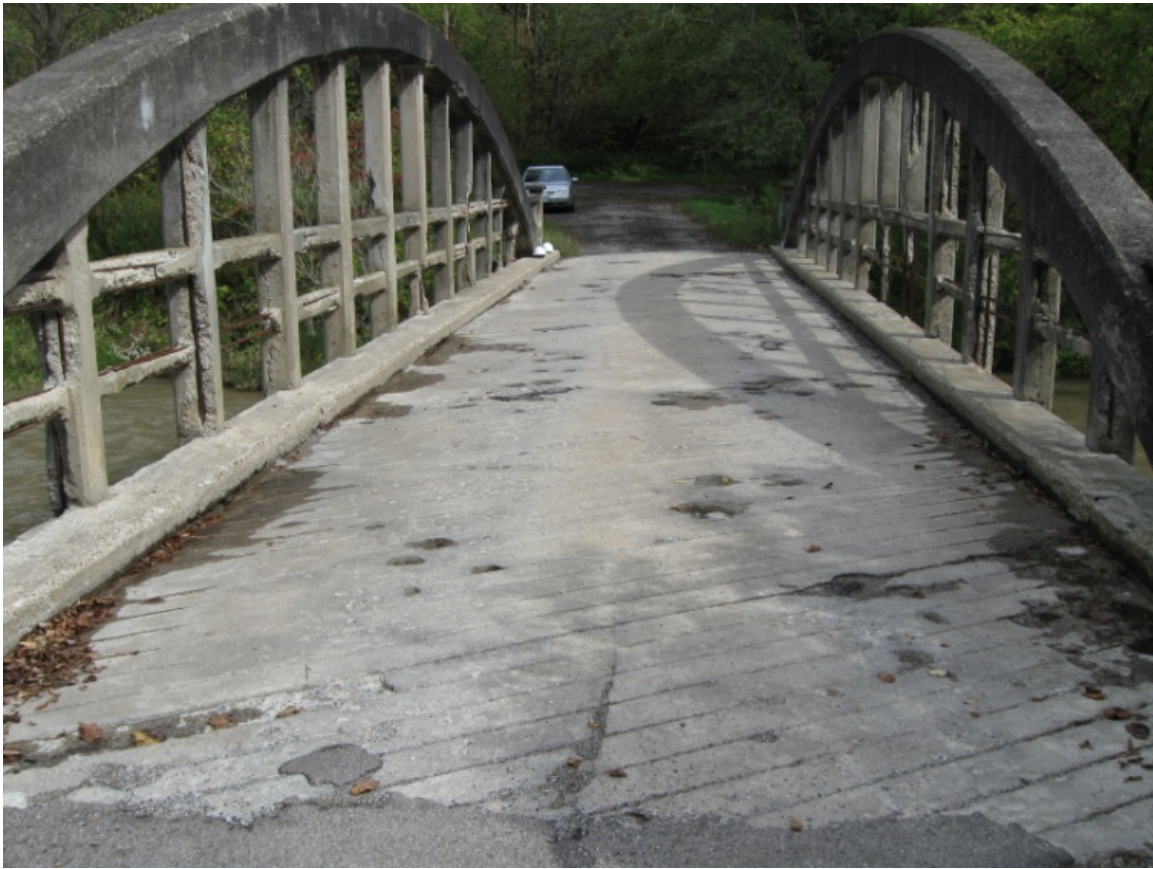
Photo 1 Bridge Deck showing cracks and potholes
