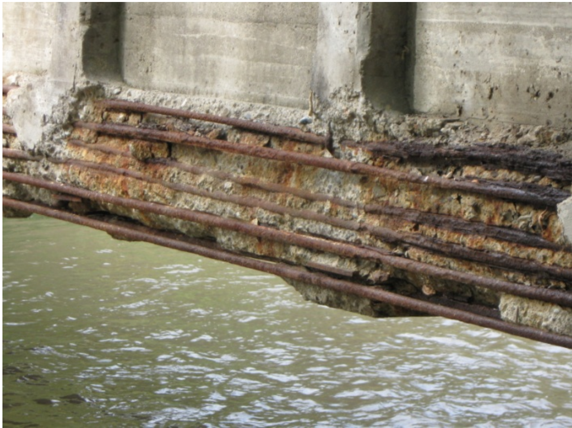
Photo 5 Truss Bottom Chord showing severe spalling
