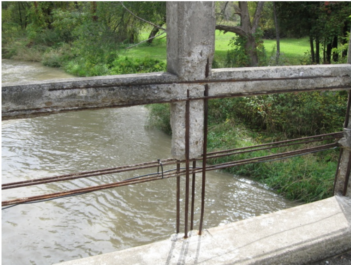
Photo 7 Vertical and Horizontal Spandrel Members showing severe spalling
