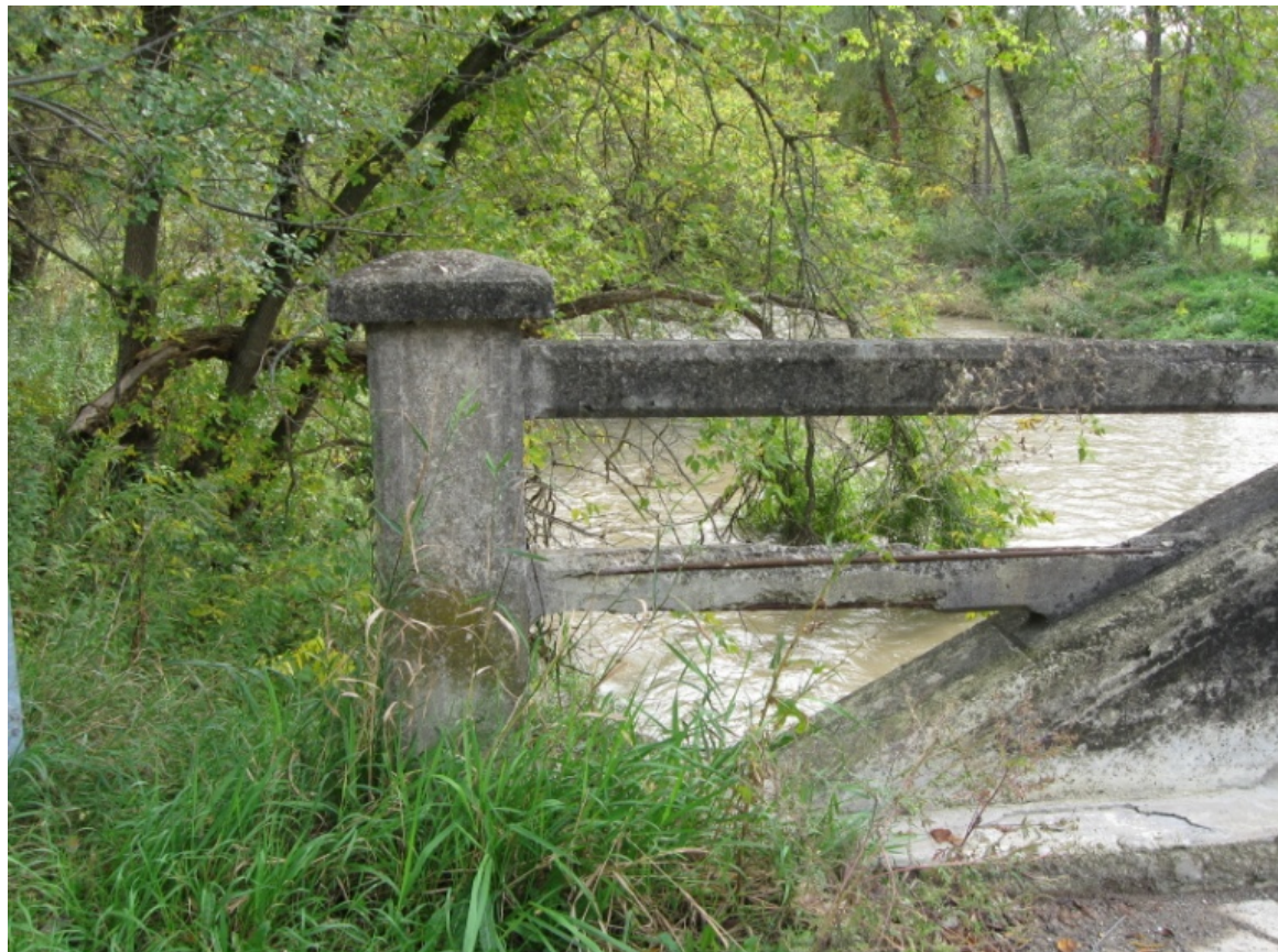
Photo 8 Handrail showing delamination
