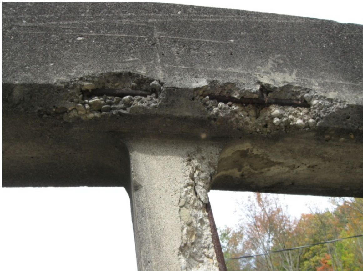
Photo 4 Truss Top Chord showing spalling
