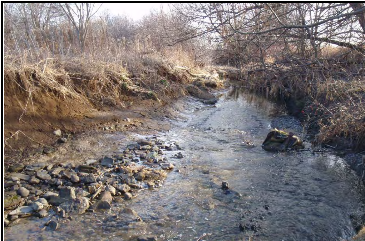
PHOTOGRAPH NO.: B8 FROM: LOOKING: COMMENT: Reach West 1 Bank erosion
