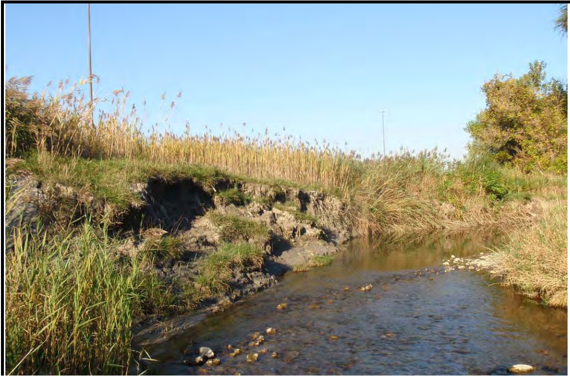
PHOTOGRAPH NO.: B3 FROM: LOOKING: Downstream COMMENT: Reach Main 1 – South side of 407
