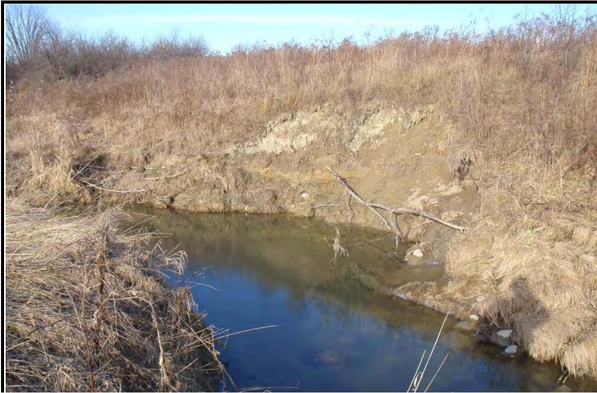
PHOTOGRAPH NO.: B9 FROM: Channel LOOKING: Upstream COMMENT: Reach West 2 Bank Erosion
