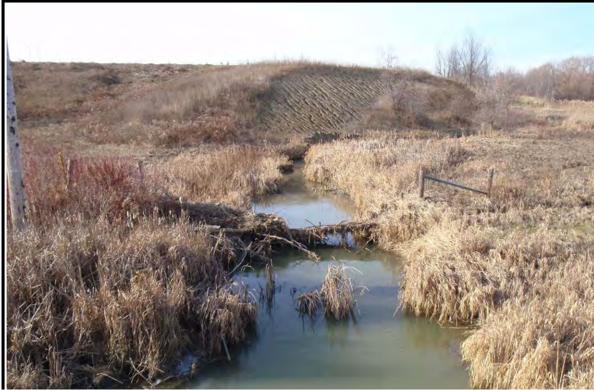
PHOTOGRAPH NO.: B7 FROM: Channel LOOKING: Upstream at eroding west bank COMMENT: Reach West 1
