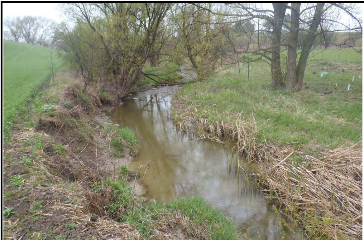
PHOTOGRAPH NO.: B14 FROM: LOOKING: COMMENT: Reach East 4 – Note localized bank erosion at outside bends
